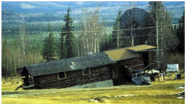
Figure 20. Leaning buildings are a characteristic of thawing permafrost in Fairbanks, Alaska.
